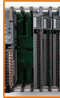
Remove existing controller cards
