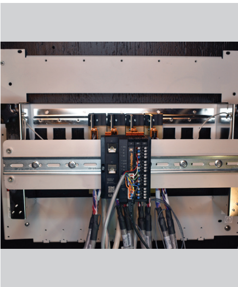
Completed and migrated DCS system
