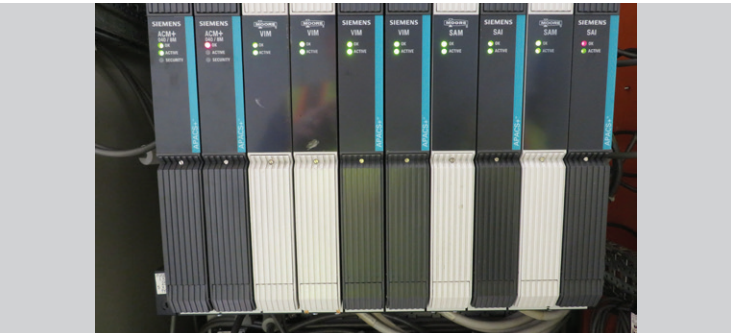
Existing Siemens Moore APACS system
