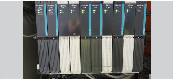
Existing Siemens Moore APACS system
