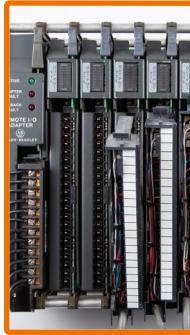
Remove existing Field Wiring adaptors
