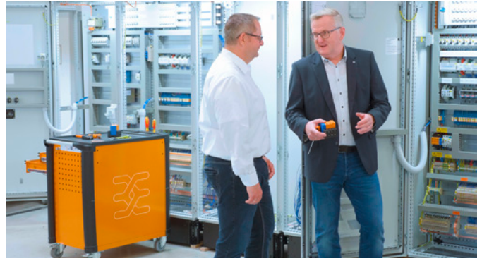
Dirk Späte, team manager for control panel building production at Bosch Building Automation GmbH, and Ralf Dolle, sales engineer at Weidmüller, are equally enthusiastic about the reliability of the VARITECTOR AC product range.
