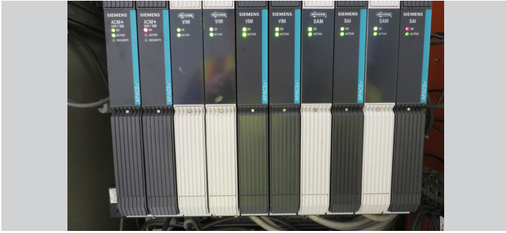
Existing Siemens Moore APACS system
